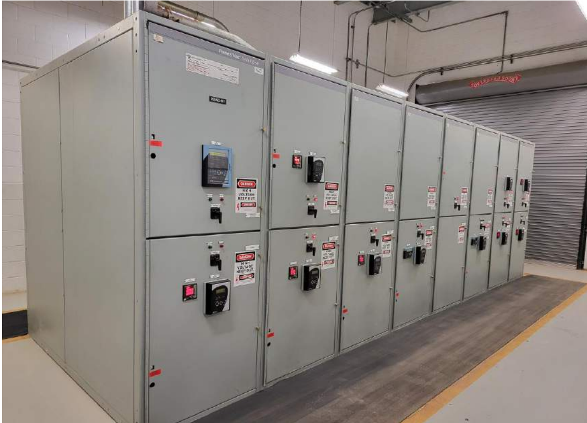
Figure 18-5: Site switchgear with two reserves
