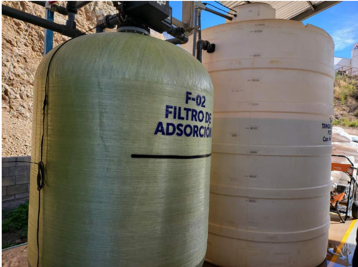
Figure 18-9: Arsenic removal tanks
