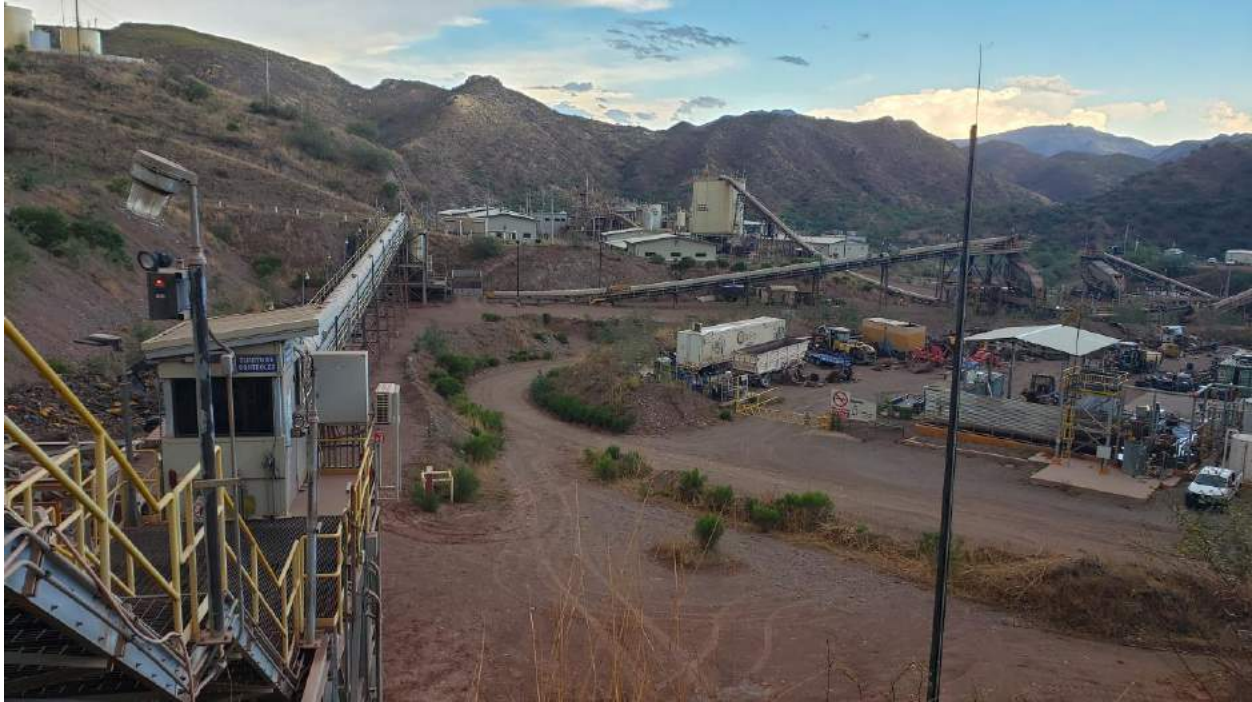
Figure 12-3: General view of the crushing facility and process plant
