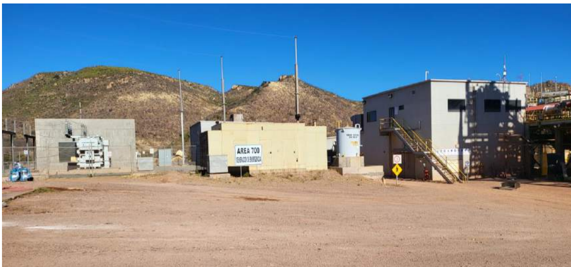
Figure 18-6: Diesel backup generator
